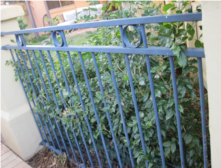
Acceptable – Vegetation unable to support the weight of a young child. May need to be monitored if the tree grows.
